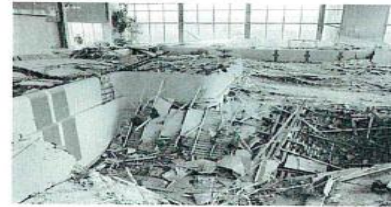
Figure 2: 9 May 1985, collapse of roof elements and ceiling during opening time of the swimming pool in Uster, Switzerland. Twelve people were killed and 19 were injured. The collapse was caused by environmental cracking of stainless steel elements in the roof construction.
