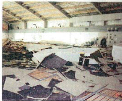
Figure 1: 1 June 2001, the morning after the collapse of ceiling and air channel in the indoor swimming pool at Steenwijk (NL). The collapse was caused by environmental cracking of stainless steel threaded bars. (Photo courtesy: Steenwijkerland municipal).
