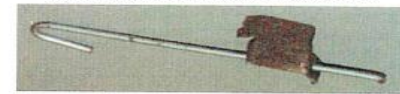
Figure 4: Completely rusted ceiling hanger after 6 years of use. The sheet was not coated, or had been provided with only a minor black organic coating. Officially such hangers are not allowed for swimming pools, but only suitable for dry buildings such as offices.
